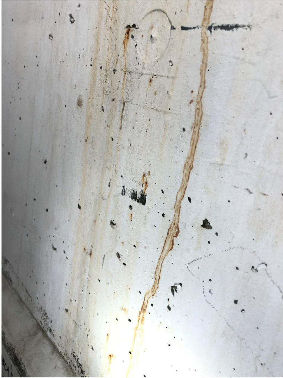
T2 leak pictures Aug 08 2023
