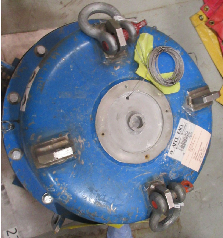
Figure 1: Small lid cap removed from F-308 exposing coiled cable - no obvious issues observed
