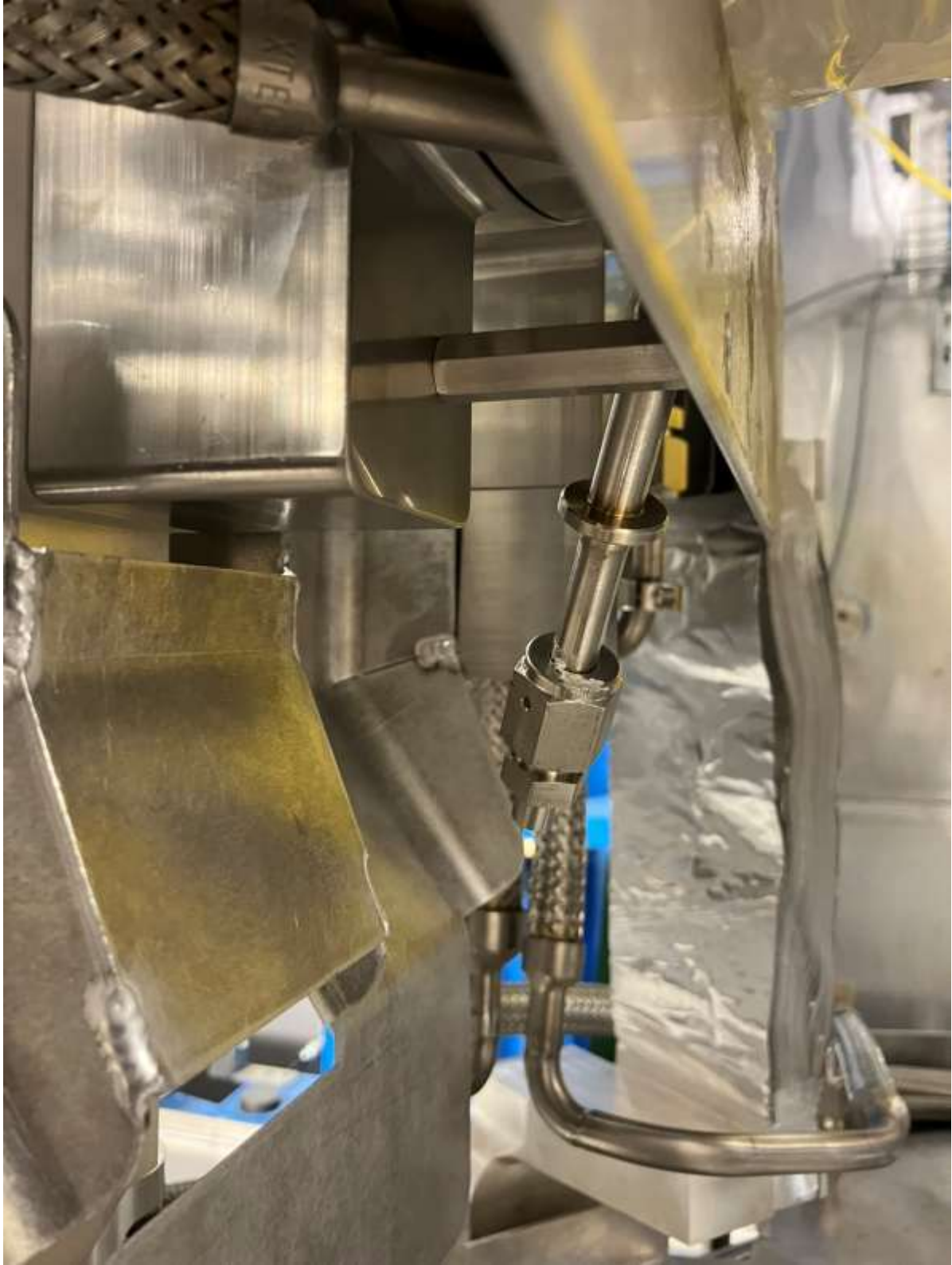
Catch spot for gas lines behind HV shielding when being fed in again.
