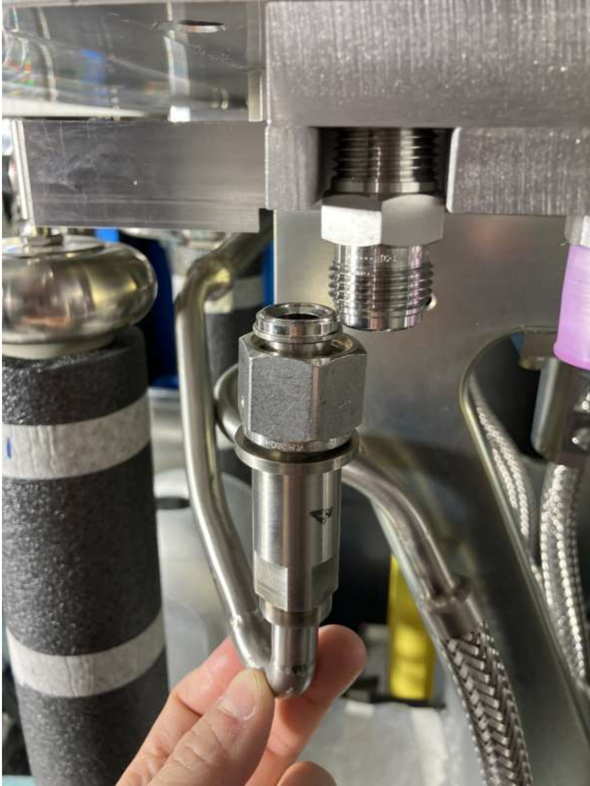
Confirmed interference between tubes on upper VCR joints
