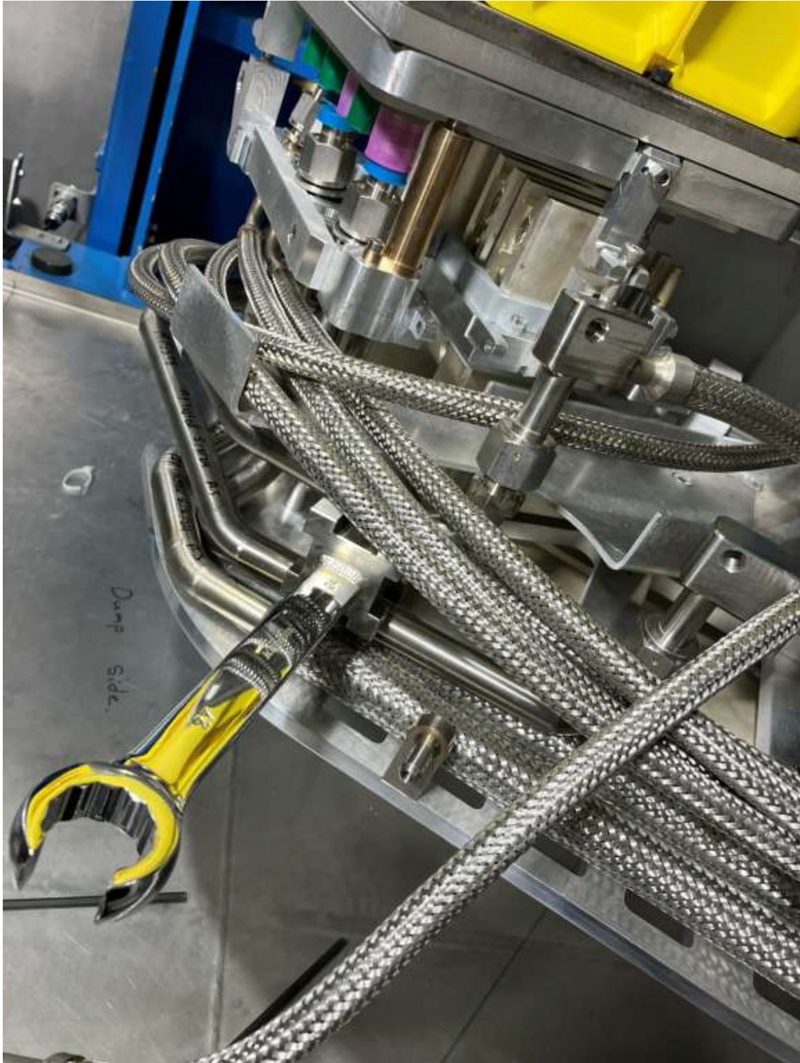
Using big handle wrench worked well to prop up the welded tube section for access to redo the joints.
