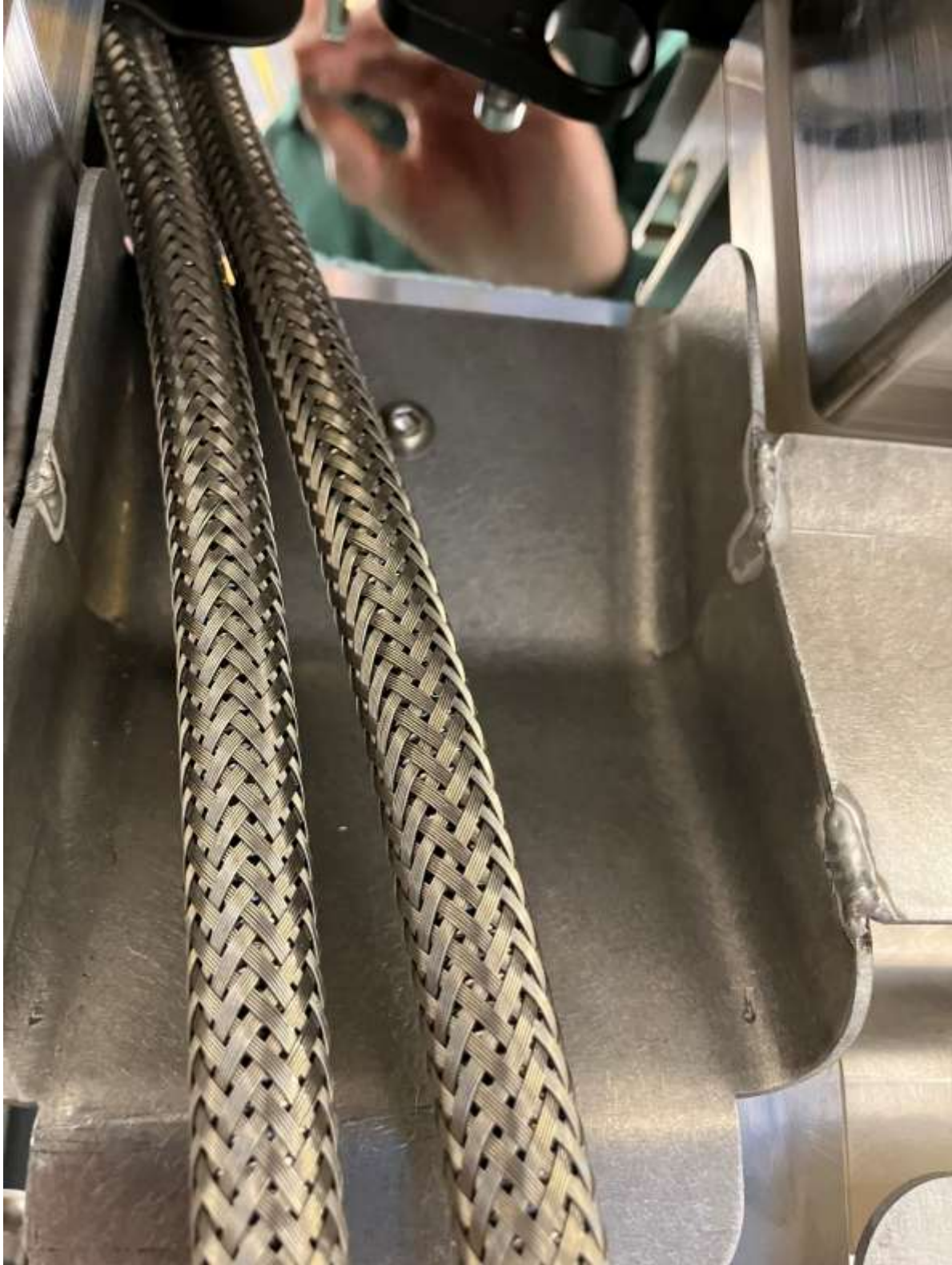
The full length of gas lines could be 'fished out' from this opening on the FE services plate.
