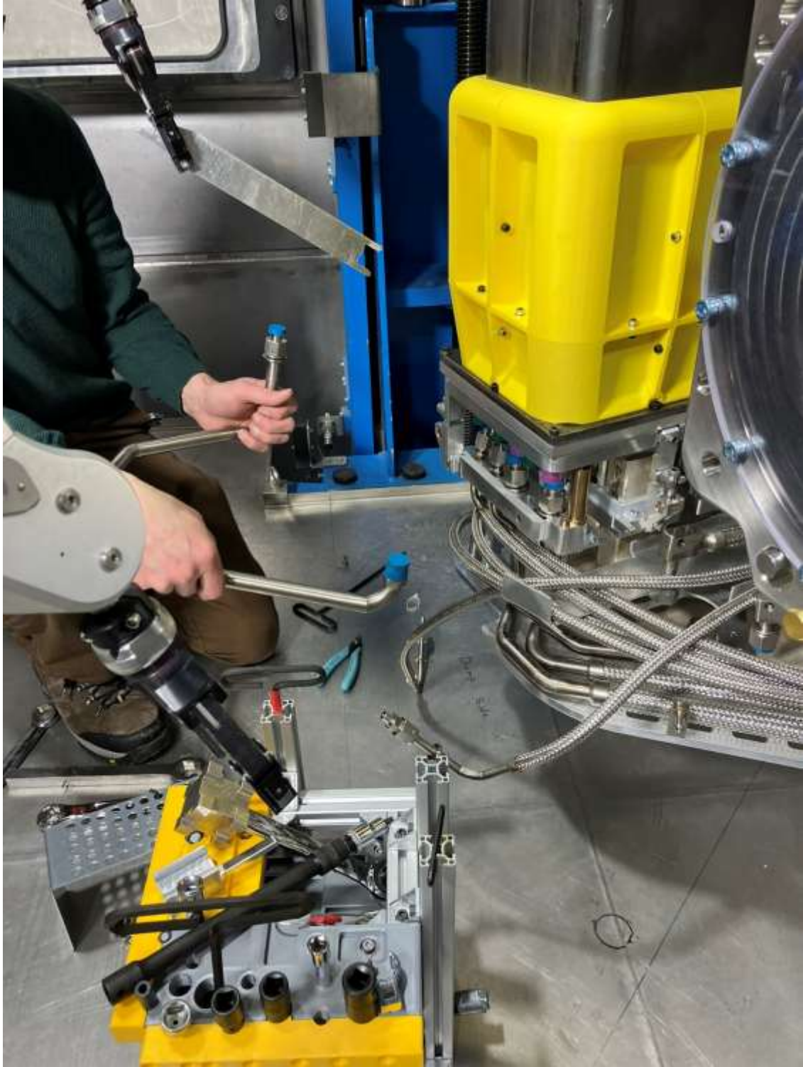
Hard line tube section looks like it can be removed without issue, tested by hand.
