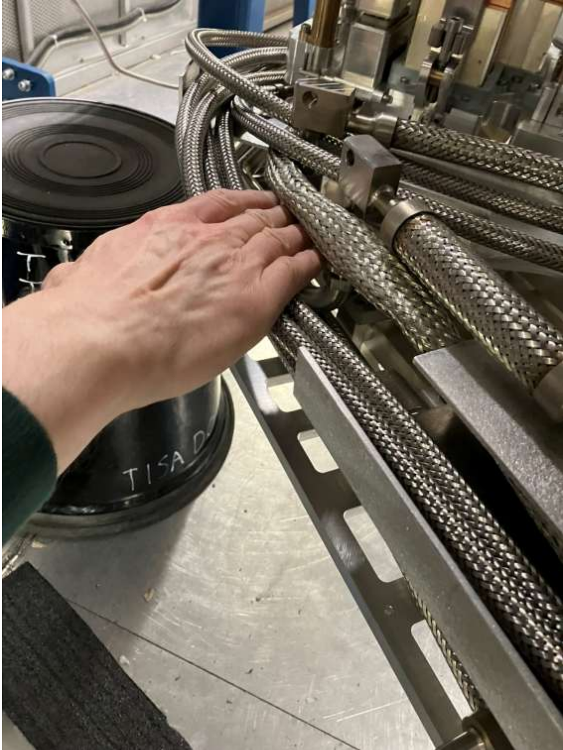
Multi-pin bundle line on AETE in TISA room interferes with access to intermediate VCR joints.
