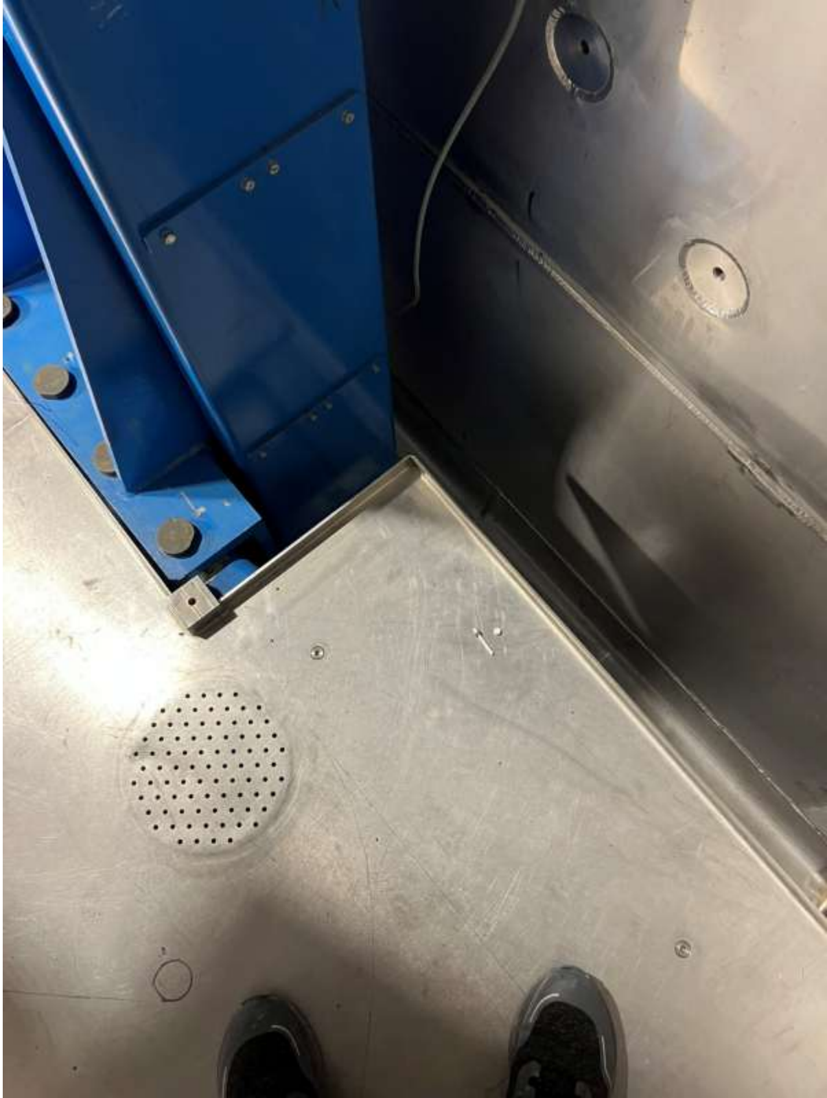
A ceramic screw broke from a dropped wrench when we first undid the top most water line's VCR joint.
