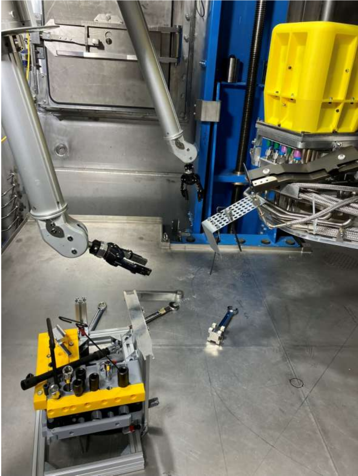
'makeshift' tool tray setup to return the busbar, camera battery died but busbar was successfully returned
