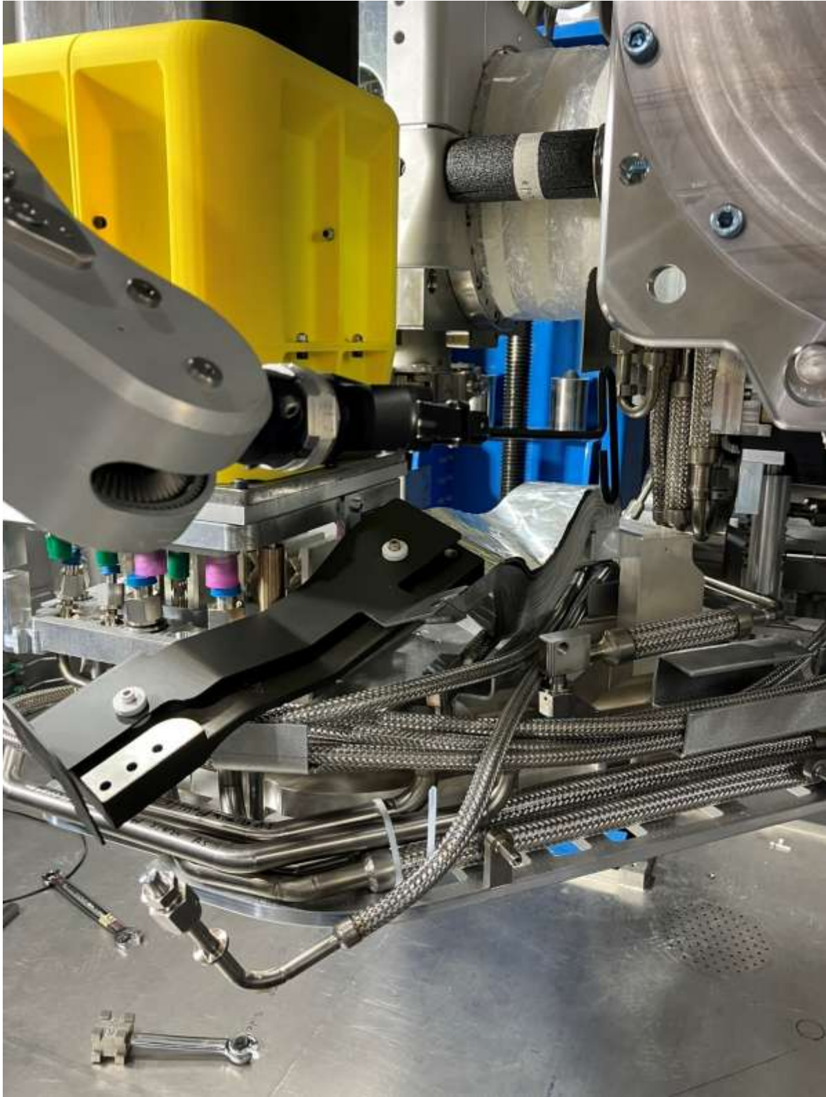
Standard T-handle tool not sufficient to access VCR joint on top most water line for positioning (butts up against HVFT).
