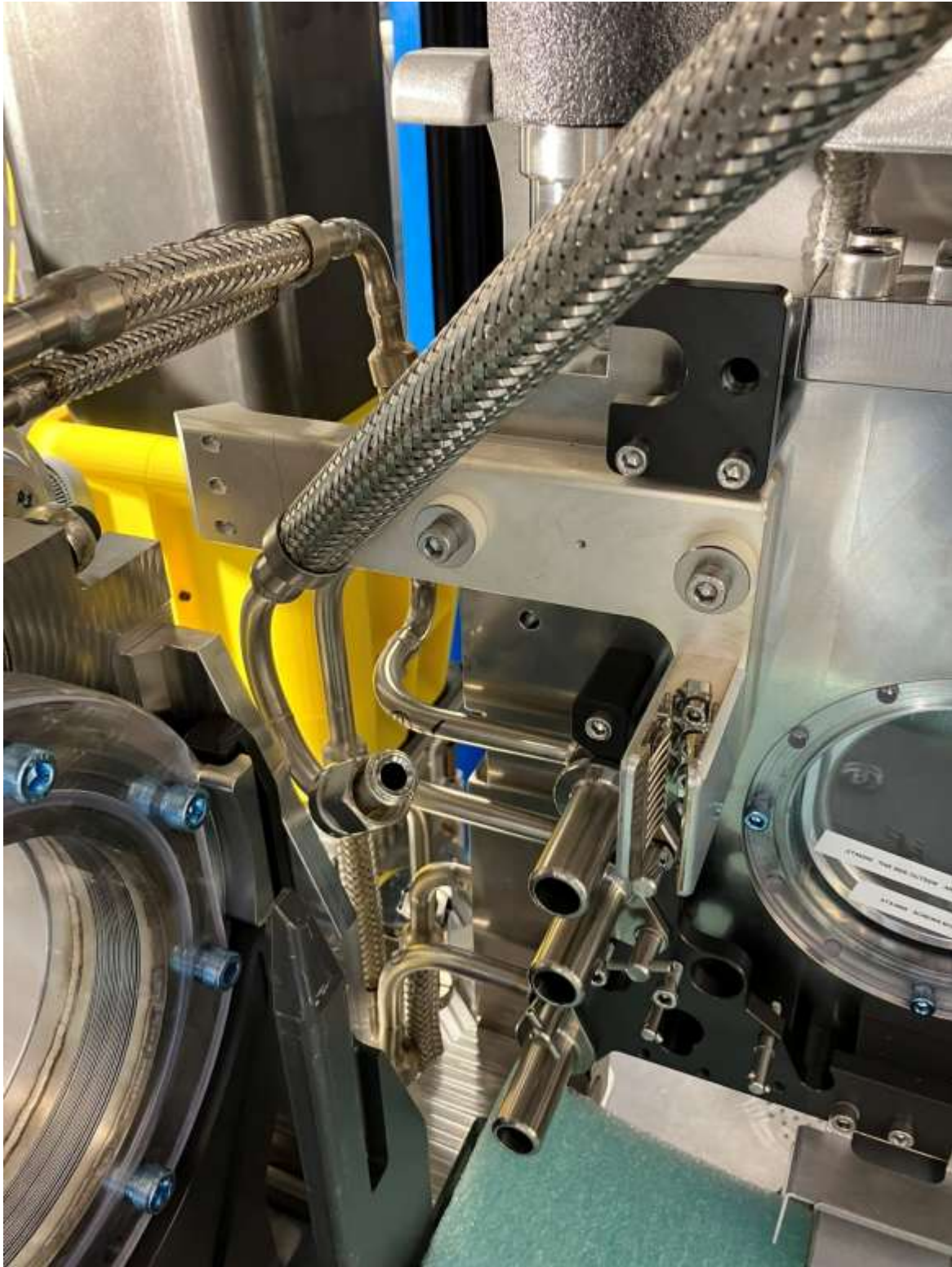
Top most VCR line could be removed and returned with the busbar out, while clamp is still on.
