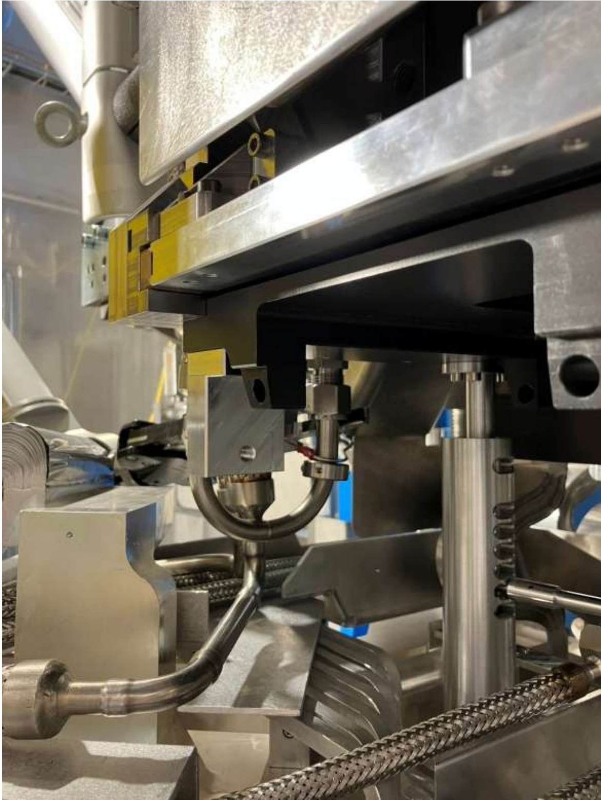
Testing the use of a hook to position VCR joint on top most water line
