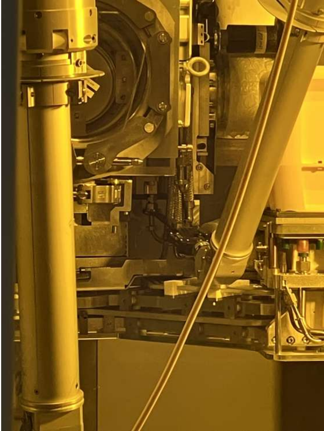
Illustration of how 'deep' the VCR joint on the top most water line is, as viewed from the hot cell window.
