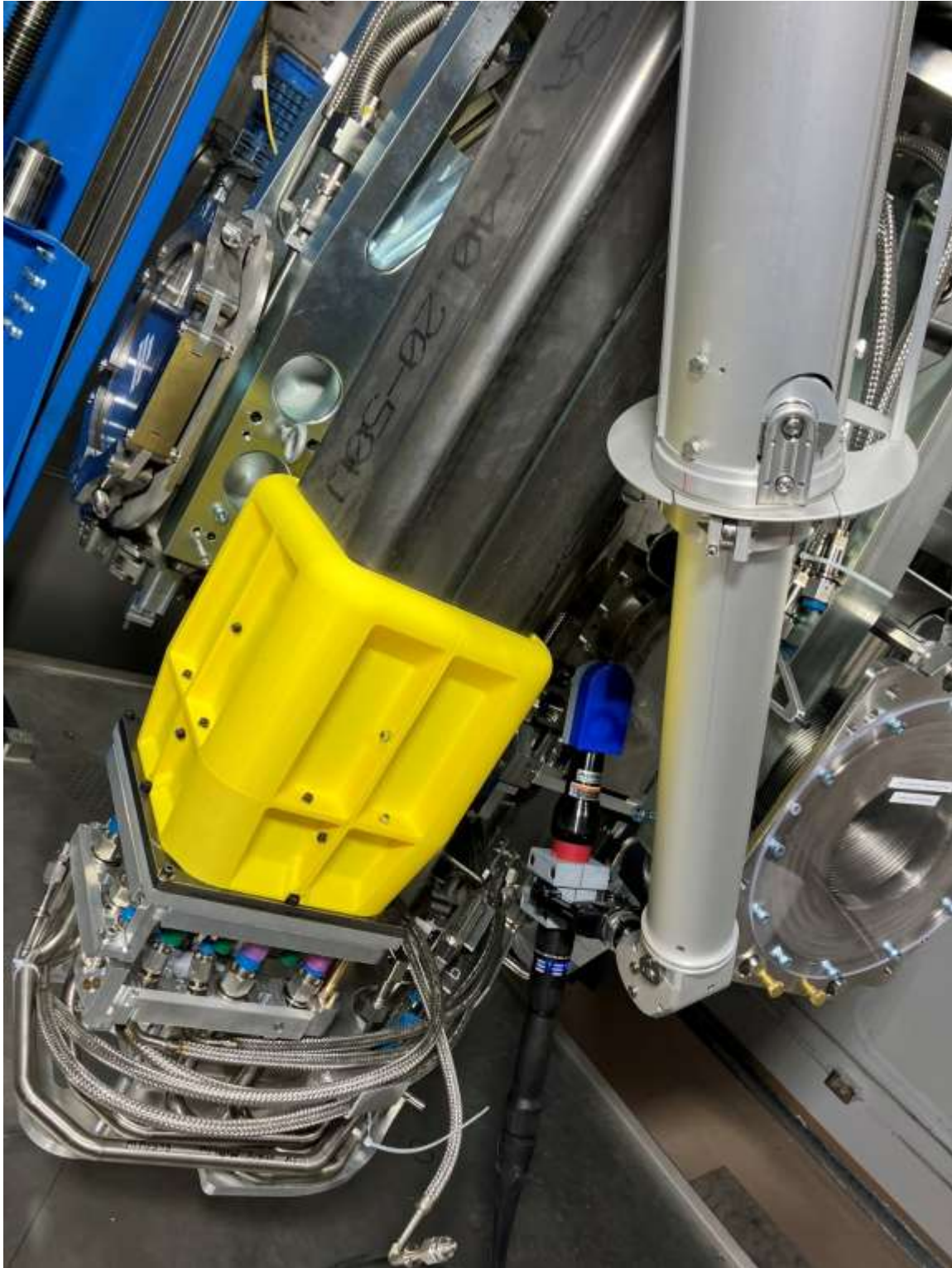
Difficulty getting torque tool to access big screw due to clearance limitations
