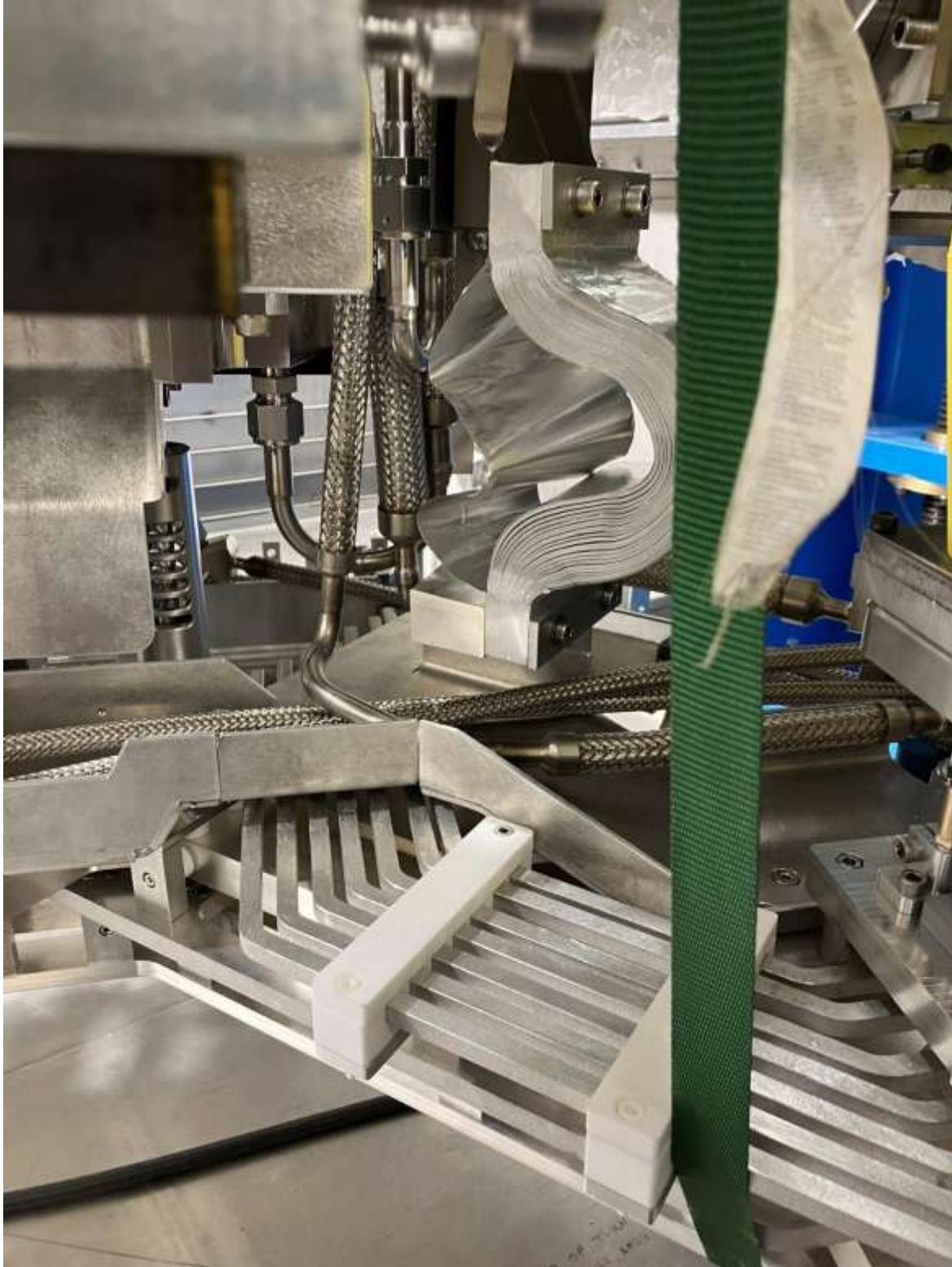
Flexible aluminum sheet conductor was found like this after manually returning the busbar (in person). In the future, we should keep in mind to check this and 'tidy' it if needed.
