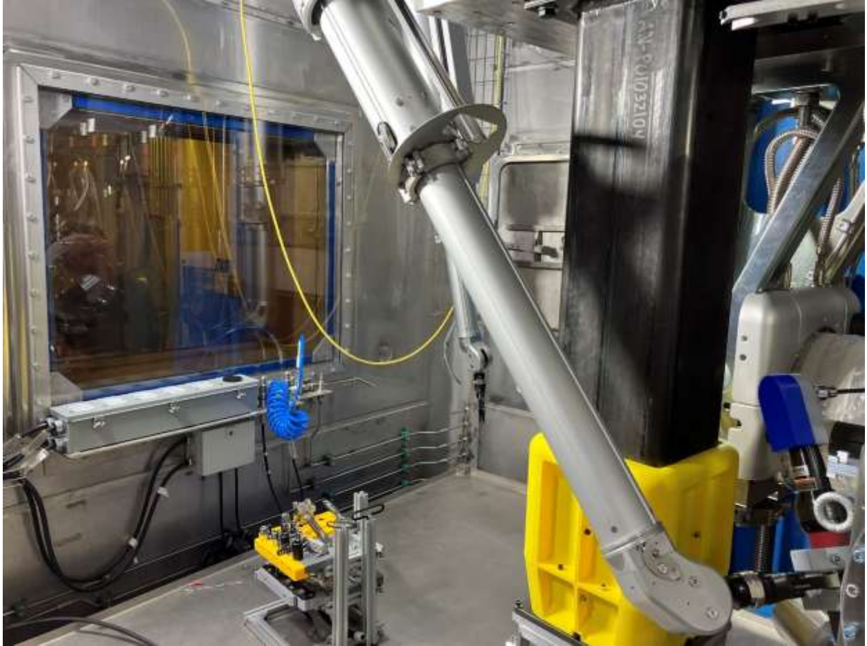
Accessing top three screws on busbar
