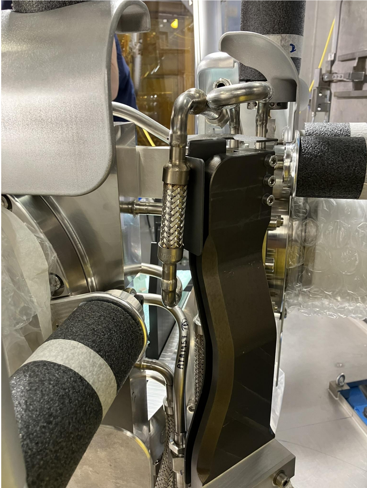
Interference of second top most line against busbar, prevents exchange.
